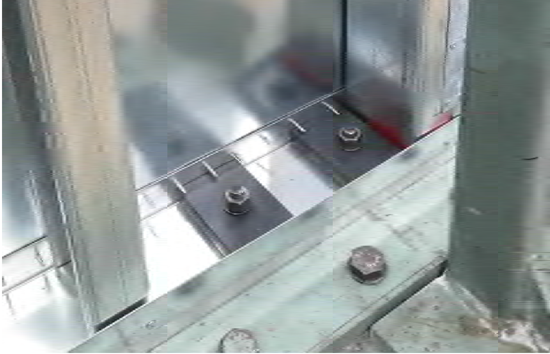
Figure B-5 Double-sheathed configuration: steel plates at shear anchors position (photo taken prior to installation of second sheathing member)
