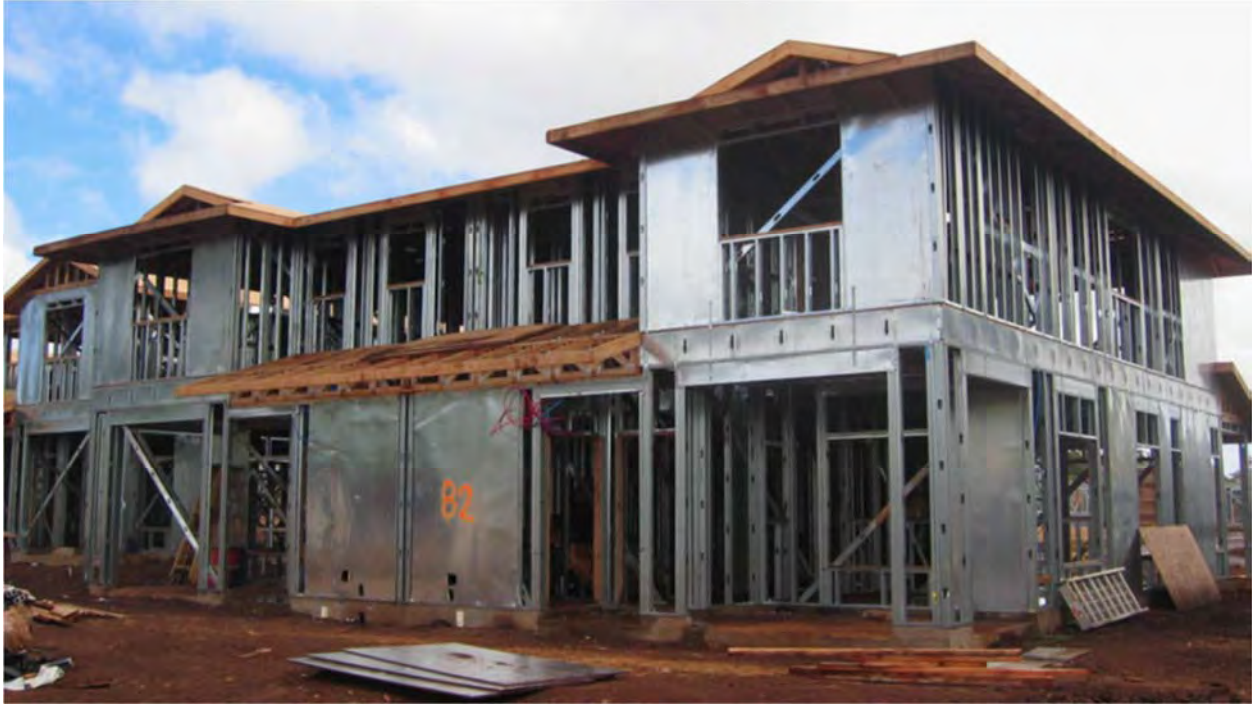
Figure 1.1 Cold-formed steel used as structural members and cladding for a house using CFS shear walls as SFRS (photo courtesy of J. Ellis, Simpson Strong-Tie Co. Inc.)
