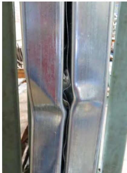
Figure 3.14 Built-up chord studs split due to out-of-plane forces caused by shear buckling of the sheathing
