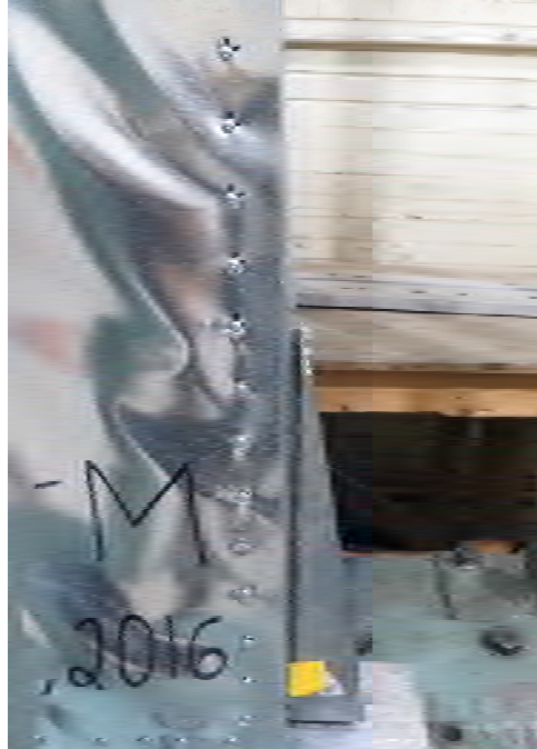
Figure 3.12: Double-sheathed chord stud web damage at holdown location.
