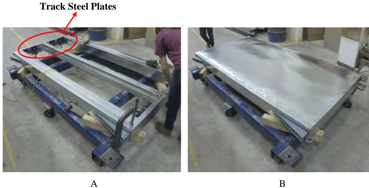
Figure 2.14: Assembly of a double-sheathed wall. A) Installation of field stud and track steel plates. B) Installed sheathing panel.
