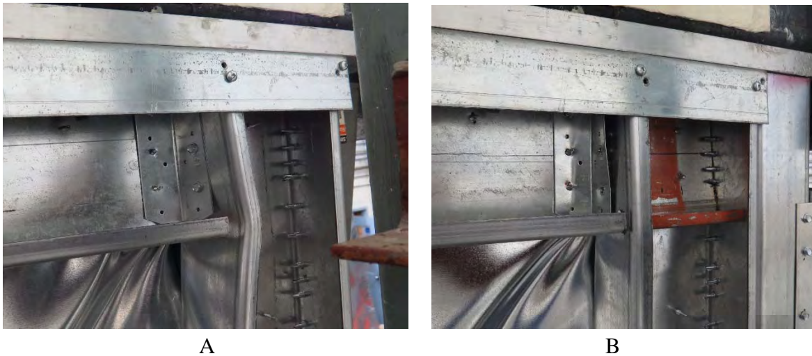
Figure 3.13: Chord stud flange damage at corners. A) Before installing stiffeners. B) After installing stiffeners.
