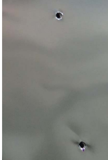
Figure 3.4: Pull-through failure of a field stud connection from out-of-plane forces.
