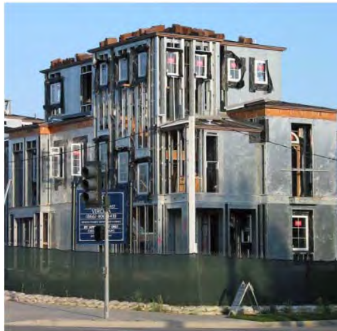
Figure 1.2: Typical residential cold-formed steel framing using cold-formed steel sheathed shear walls (photo courtesy of Jeff Ellis, Simpson Strong-Tie Co. Inc.).
