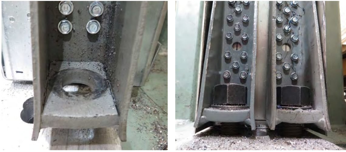
Figure 3.15: A) Single holddown plate damage. B) Double holddown plate damage.
