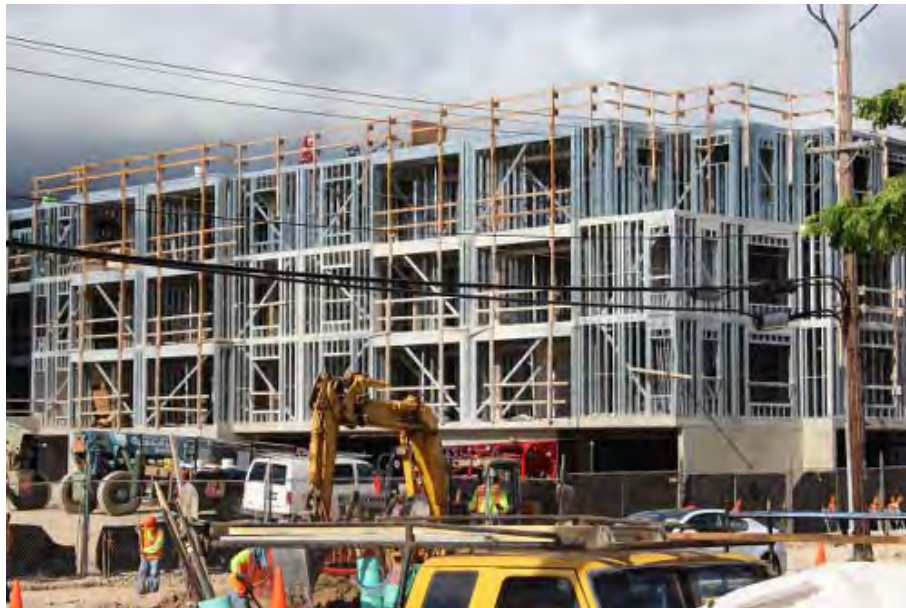
Figure 1.1: Cold-formed steel framing used in the construction of a mid-rise building in Pearl City Hawaii, (Hawaii Steel Alliance, (2017)).
