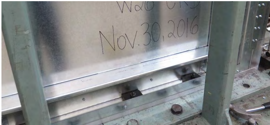
Figure 2.18: Placement of steel plates inside the flanges of the bottom horizontal framing member.
