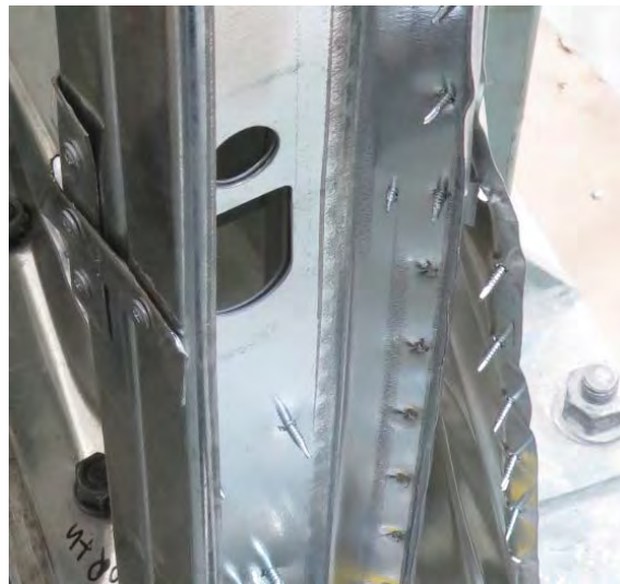
Figure 2.15 Sheathing screw pull-out failure
