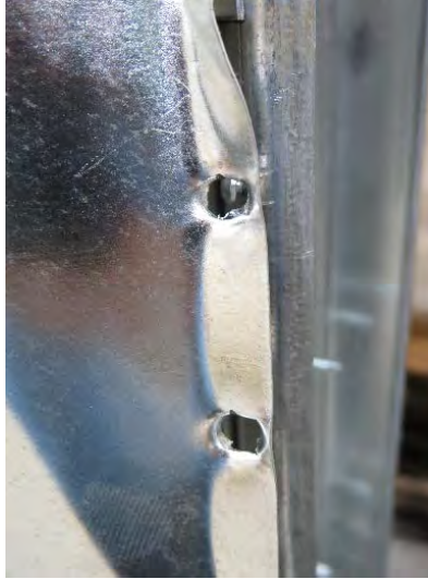
Figure 2.16 Screw pull-through sheathing failure
