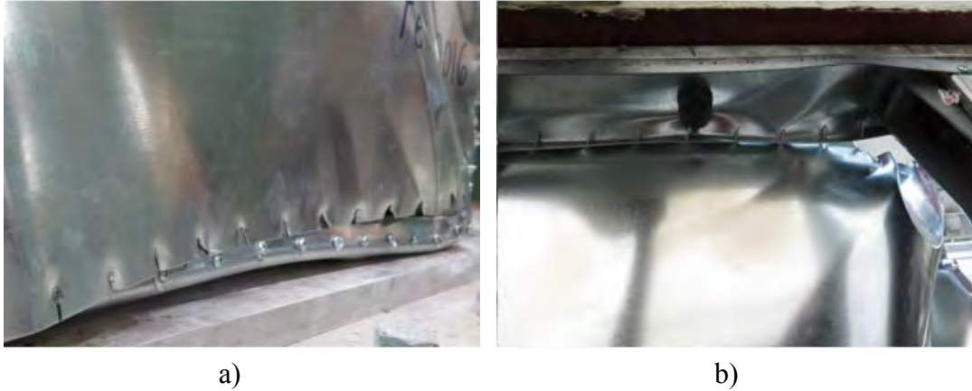
Figure 2.22 a) Deformation and uplift of bottom track, b) Deformation and uplift of top track
