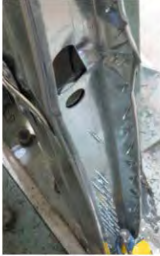
Figure 2.23 Local Buckling of the chord studs in 610×2440mm (2'×8') walls
