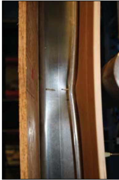
(b) detail of (a) at point of lateral load application, connection damage limited
