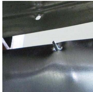
Figure 2.15 Sheathing Screw Pull-out Failure
