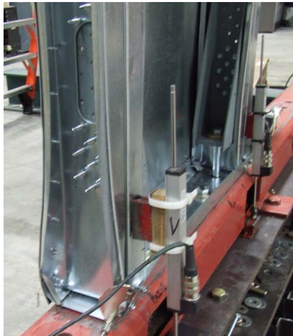
Figure 15 Local buckling of boundary studs of 27-mil sheet steel shear wall
