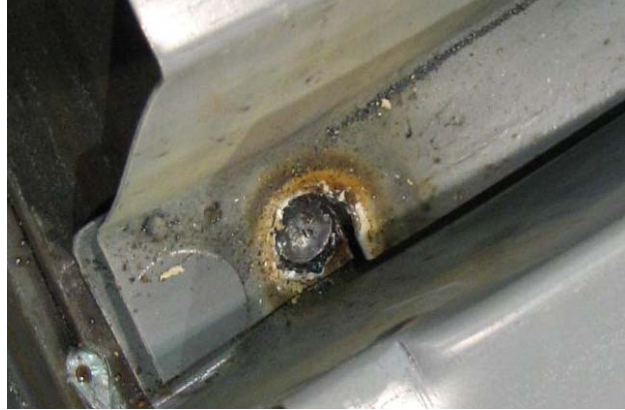
Figure 4-8: Weld Crack from Diaphragm Loading
