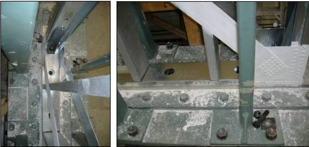
Figure 2.41 Corner detail of specimen 46 A-C
