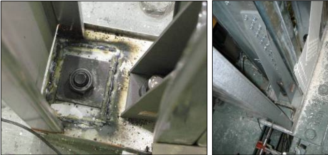
Figure 2.37 Corner detail of specimen 30 A-C
