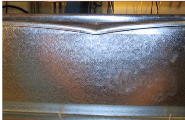
(b) Beam buckled
