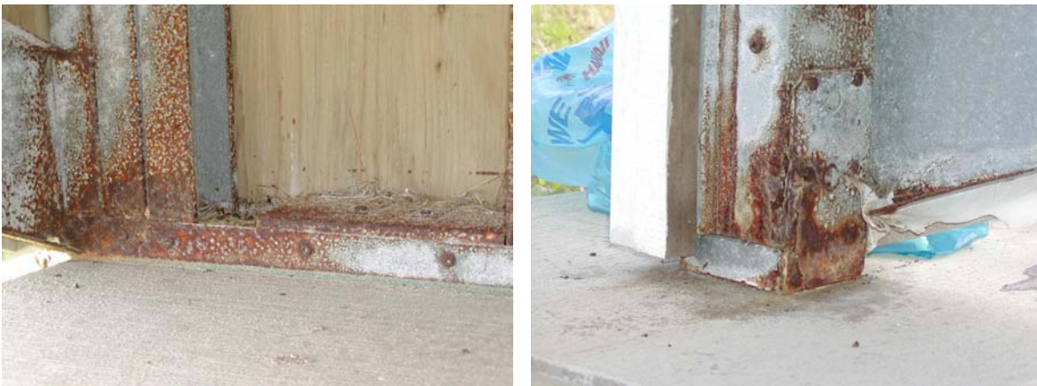
Figure 7.31: Crawl space cripple wall and post, MCBH Coastal after 28 months.
