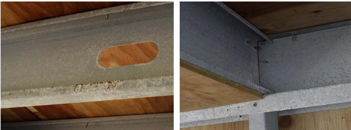
Figure 7.32: Crawl space exposed floor joists, MCBH Coastal after 5 months.
