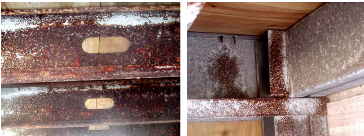
Figure 7.36: Crawl space exposed floor joists, MCBH Coastal after 21 months.
