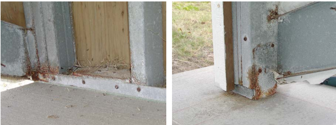
Figure 7.29: Crawl space cripple wall and post, MCBH Coastal after 16 months.
