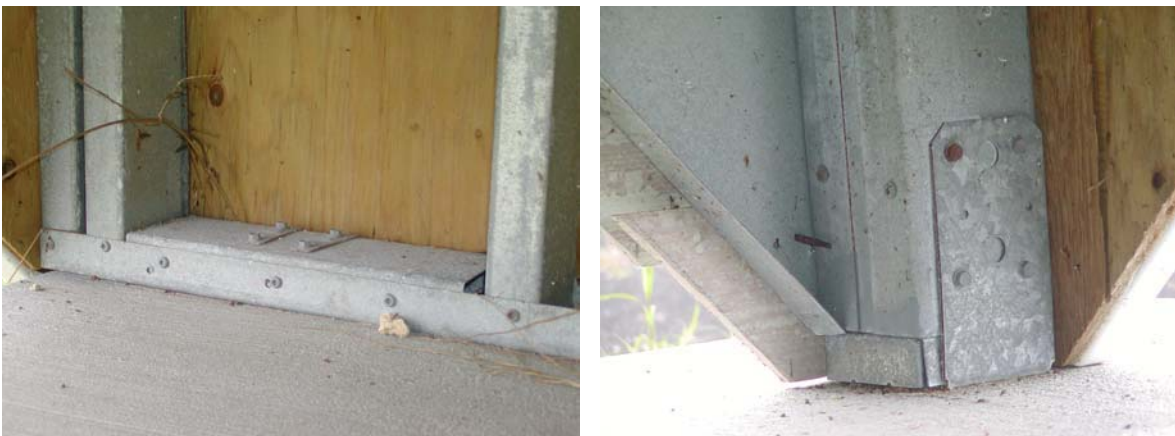
Figure 7.12: Crawl space cripple wall and post at MCBH Inland after 28 months exposure.
