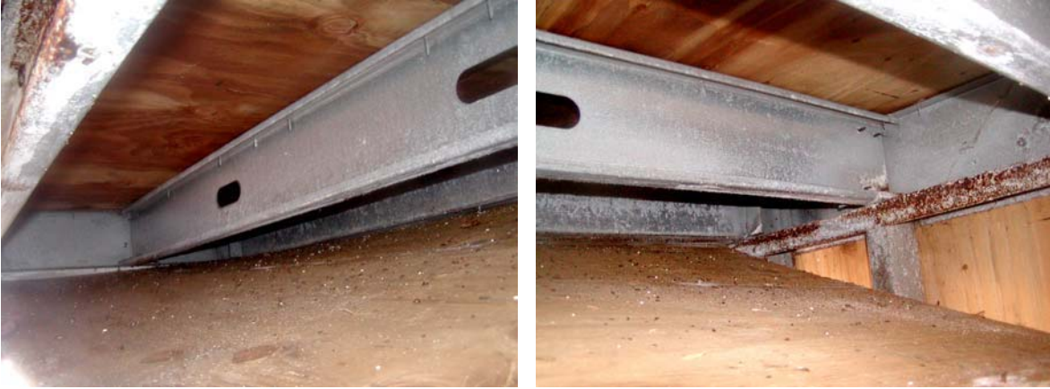
Figure 7.37: Crawl space covered floor joists, MCBH Coastal after 21 months.
