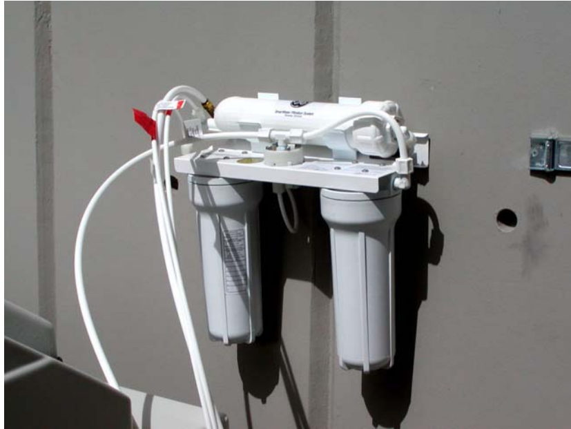
Figure 5.4: Reverse Osmosis water purifier behind the QFOG chamber
