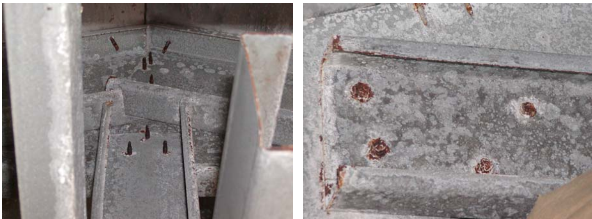
Figure 7.27: Vented attic framing at MCBH Coastal after 28 months.
