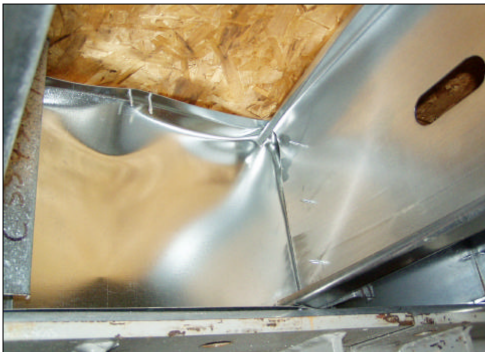
Figure 5.3: Photograph of a Punch-Through Failure of the OSB
