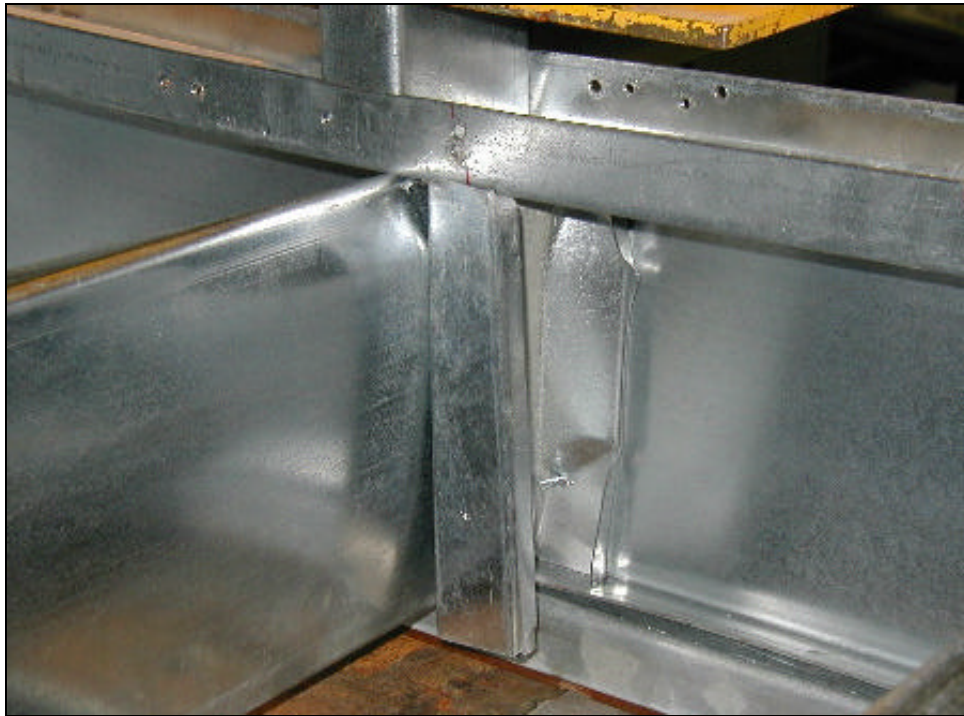
Figure 5.2: Photograph of a Stiffener Failure
