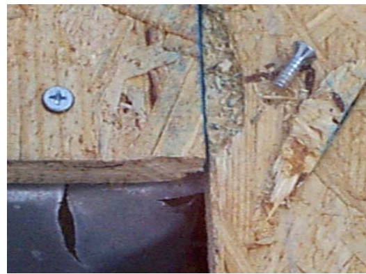
Figure 22- Fatigue failure of sheathing
