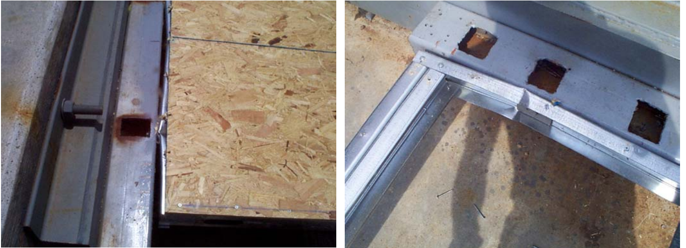
Figure 24 -Damage caused to tracks due to absence of tie-down anchors on end studs
