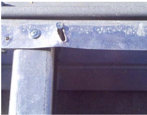
Figure 21- flaring of steel track
