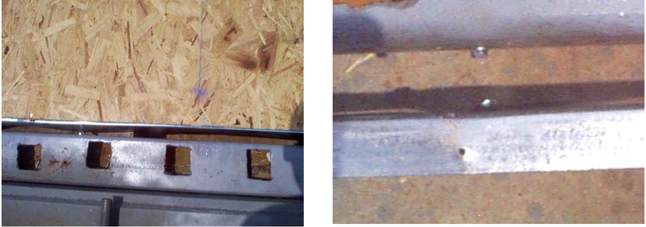
Figure 27- Separation of wall track from steel distribution beam.
