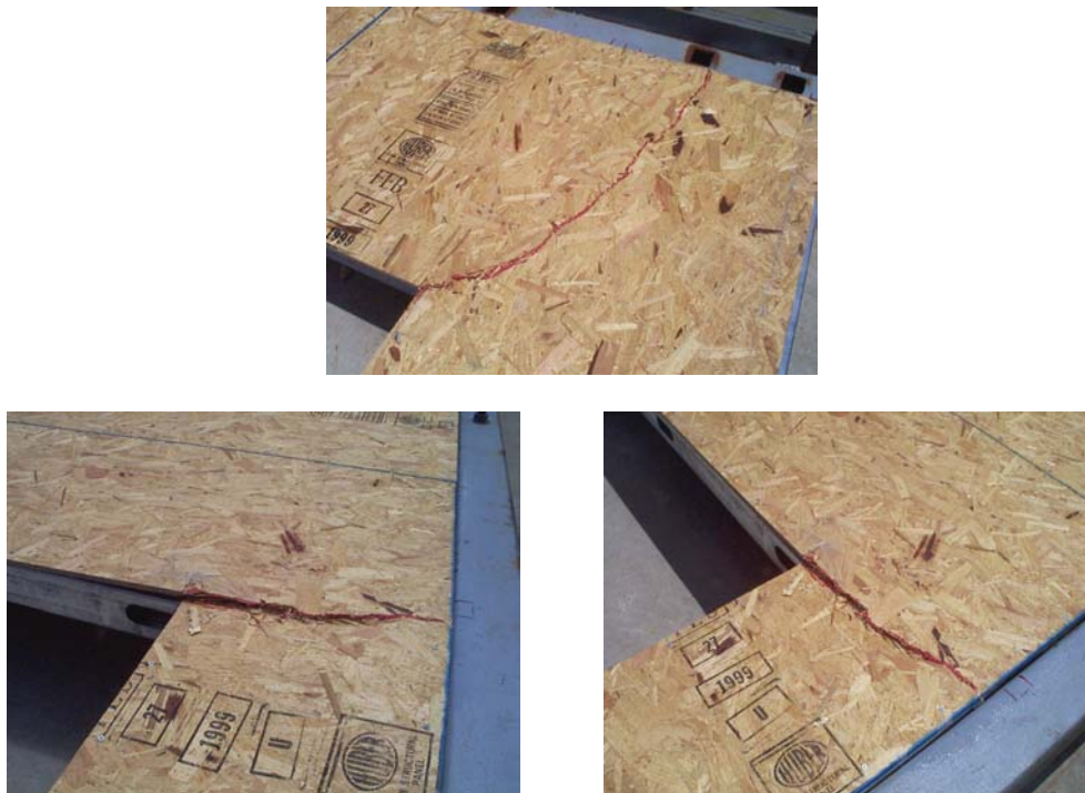
Figure 28- Failure of walls with gusseting around openings.
