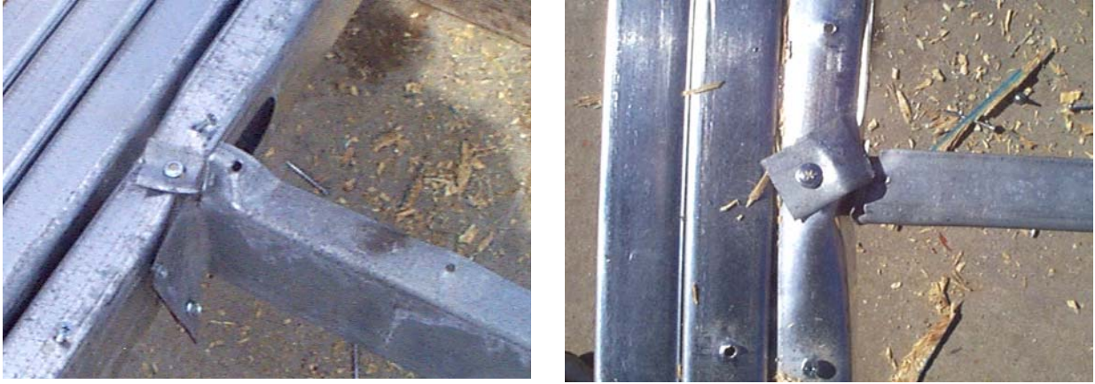
Figure 25- Tab tear failure of wall headers and track below openings.
